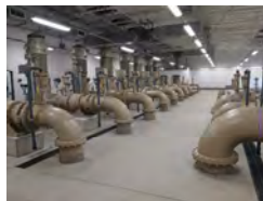
IRWD's Eastwood Recycled Water Pump Station:
