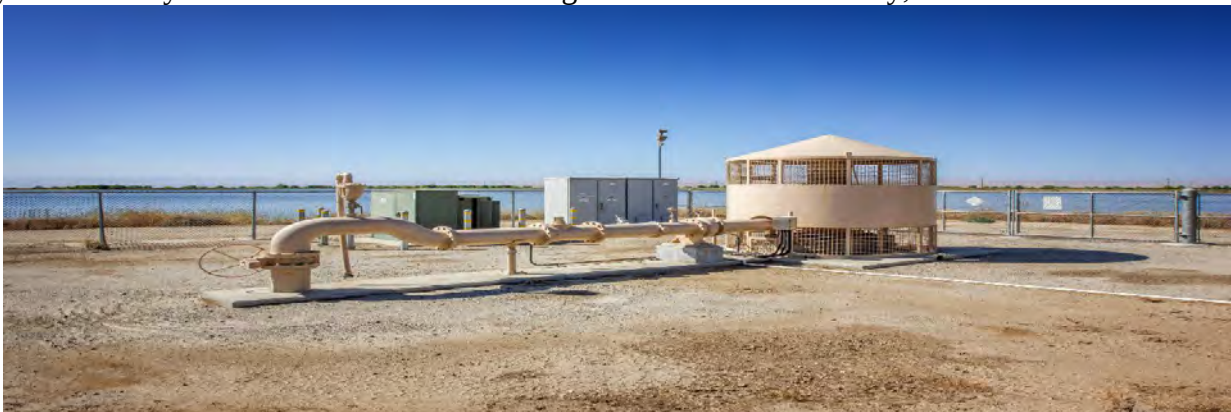
IRWD Water Banking Facility
